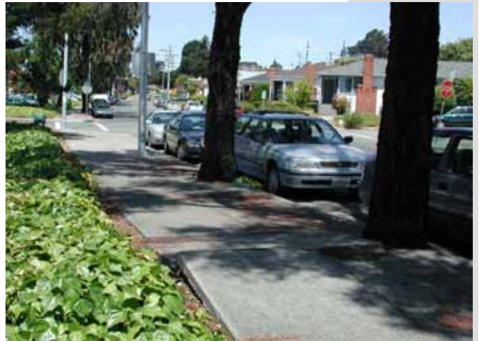
Station Area Buckled Sidewalk
