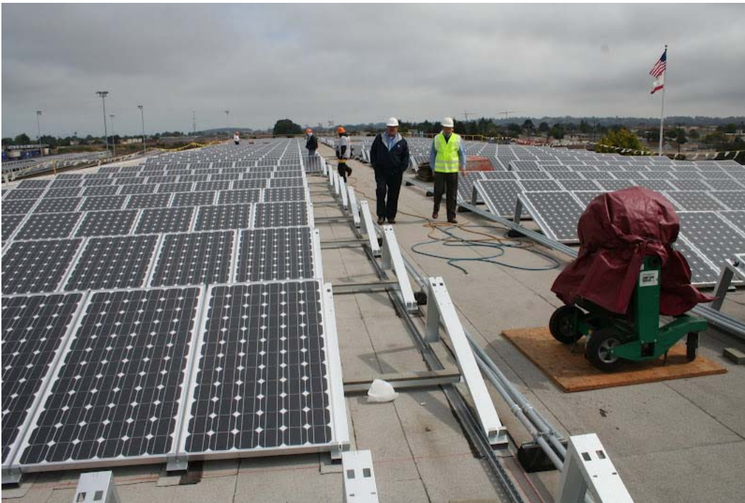
Figure E: Photos of typical photovoltaic system (BART Richmond Shop rooftop, 2012)
